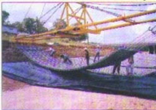
The Installation concrete mat system with a crane equipped with spreader bar.
